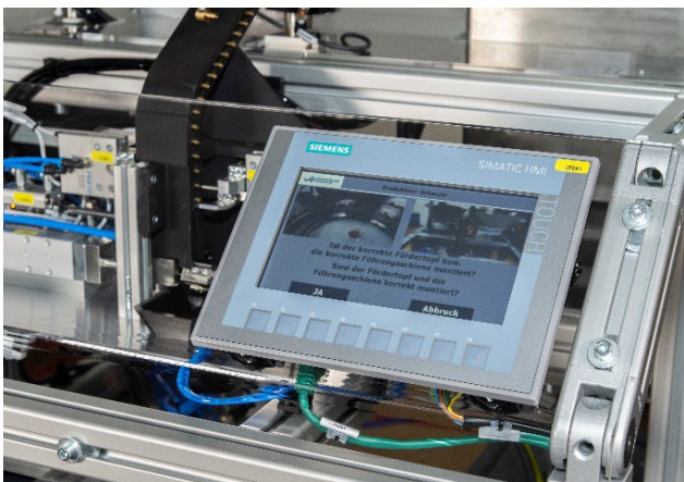
Example Siemens HMI control
