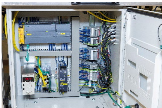
Control cabinet with integrated PLC
